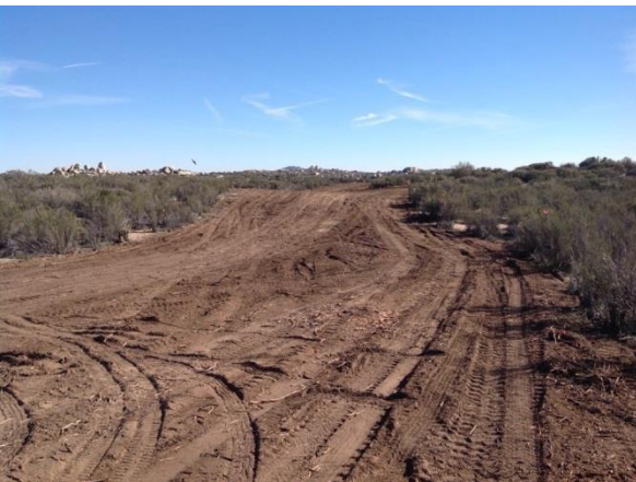
Photo 3: On 1.18.17, approximately 11,700 square feet of vegetation was mulched outside of the currently approved limits of disturbance. BLM issued a "Noncompliance" in accordance with Section 5.2 of the ECMP.
