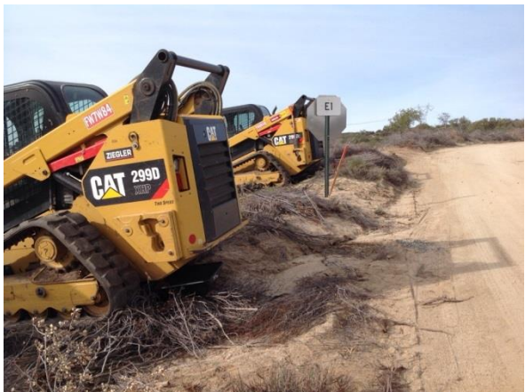
Photo 4: ECMs observed containment drip pans under parked equipment to prevent potential leaking equipment from staining soils in accordance with MM HAZ-1A and the Hazardous Materials Management Plan.
