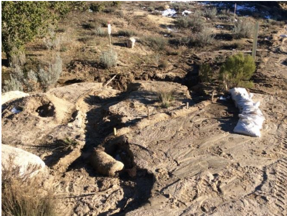
Photo 3: ECMs and SWPPP inspectors checked the project site for areas where erosion and sediment control devices were missing or failing. These issues were documented and reported to Tule Wind, LLC. During this reporting period, construction crews were onsite daily to repair, maintain, and install additional erosion and sediment control devices in accordance with MM HYD-1 and the SWPPP.
