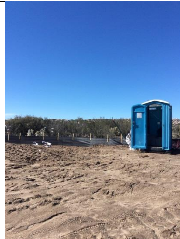
Photo 4: On Friday, 1.27.17 ECMs observed toilet paper, which had blown out of the portable sanitation facility at the H-String laydown area into nearby vegetation during the windy conditions (gusts over 40 mph). This issue has been recorded as a "Problem Area" according to Section 5.2 of the ECCMP. Biological monitors are anticipated to sweep the area to clean up all remaining litter in accordance with MM BIO-7D.
