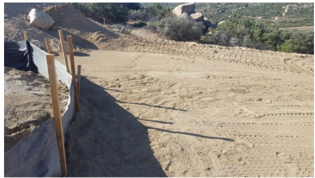
Photo 2: On April 22, ECMs confirmed that the silt fence surrounding the concrete washout basin had been repaired in accordance with Section 7.10 of the SWPPP and the concrete wash outside the basin containment had been cleaned.
