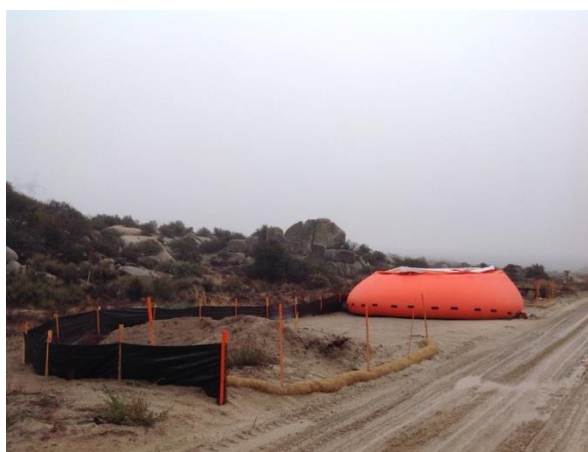
Photo 8: Temporary 10,000-gallon water tanks installed with proper erosion and sediment control devices in accordance with the Fire Prevention/Protection Plan, NTP-3, and the SWPPP.
