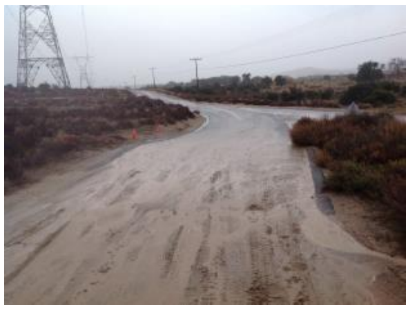
Photo 4: ECMs noted that McCain Valley Road is not properly stabilized at the paved entrance/exit in accordance with the SWPPP. Tule Wind LLC is aware of the issue and is working to stabilize the entrance/exit without impeding public access.
