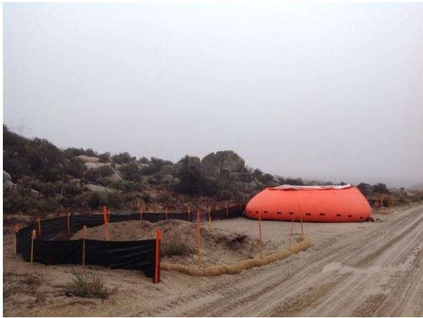
Photo 3: Temporary 10,000-gallon water tanks installed with proper erosion and sediment control devices in accordance with the Fire Prevention/Protection Plan, NTP-3, and the SWPPP.
