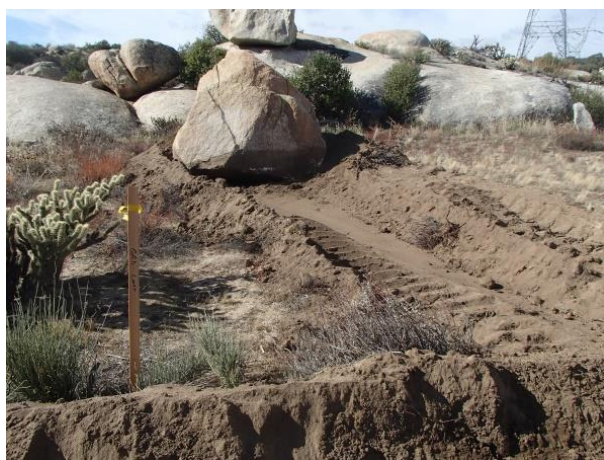
Photo 7: A boulder was pushed approximately 15 feet outside of the limits of disturbance. This event is being classified as a “Problem Area” in accordance with Section 5.2 of the ECMP .
